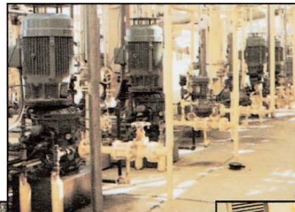
40 HP LMV-322 reactor feed pumps in southwestern refinery
